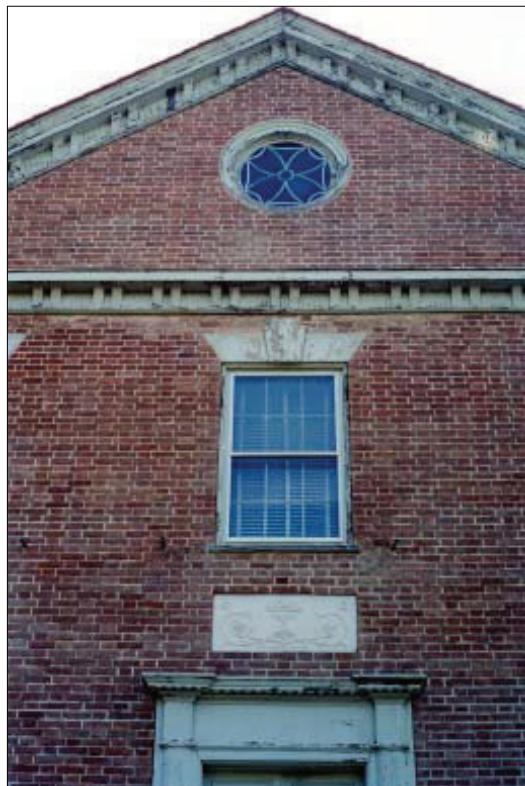
The wooden and stone details on the Teackle Mansion in Princess Anne, Somerset County, reveal a high level of craftsmanship. Exterior restoration of the property, which has already begun, will continue as funds become available. [Photo by Kip Van Blarcom]
