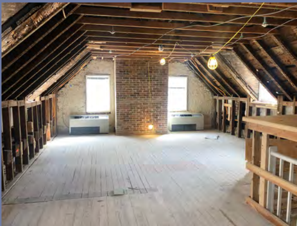
The second floor of the east wing served as living quarters for enslaved people at the Brice House. To interpret and authentically highlight this rare early living space for enslaved people, on-going work will remove 20th-century modifications while restoring the original floor level (creating a low ceiling height), stabilizing early plaster walls, and conserving the dormer windows.
