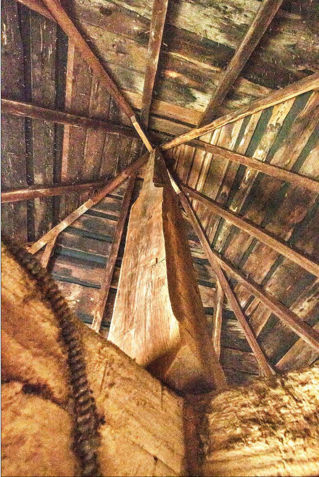
Figure 17. The smokehouse king post at La Grange, near La Plata (Willie Graham).
