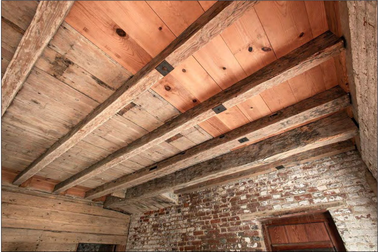
Figure 56. View of the ceiling in the main room of the workhouse/weaving house, Mulberry Fields (Willie Graham).
