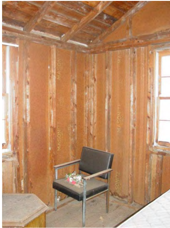
Figure VI-19: Typical Damascus cottage interior with mattress, small table, and chair. Walls are framed in 2x4s with Masonite siding. (Elizabeth Jo Lampl, Montgomery County Historic Preservation Section)
