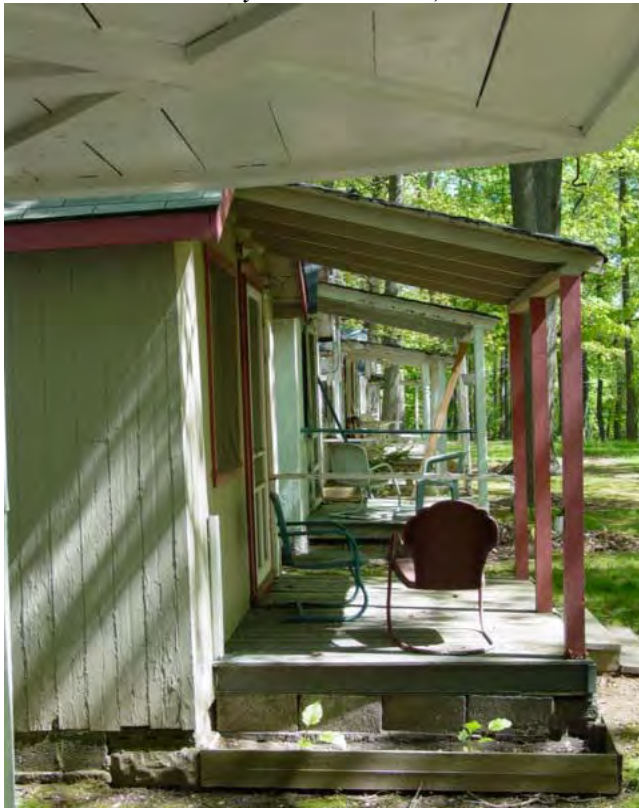
Figure VI-10: A row of porches at Spencerville Camp Meeting. (Elizabeth Jo Lampl, Montgomery County Historic Preservation Section)
