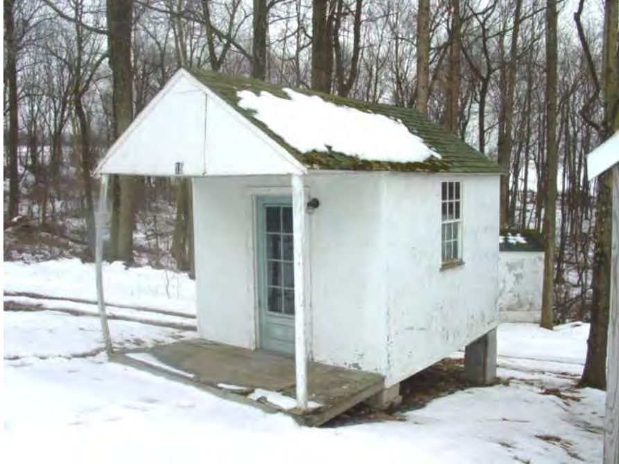
Figure VI-16: Typical Damascus camp meeting cottage walled in Masonite. (Elizabeth Jo Lampl, Montgomery County Historic Preservation Section)
