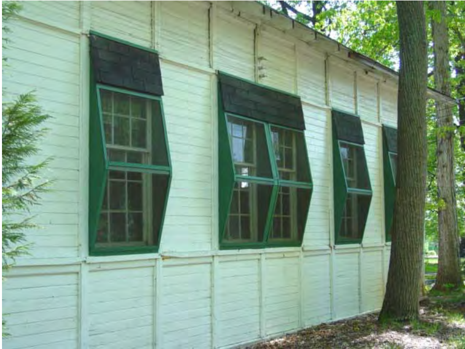
Figure VI-31: Sidewalls of the former portable schoolhouse that is today part of the dining hall at the Spencerville Camp Meeting. (Elizabeth Jo Lampl, Montgomery County Historic Preservation Section)
