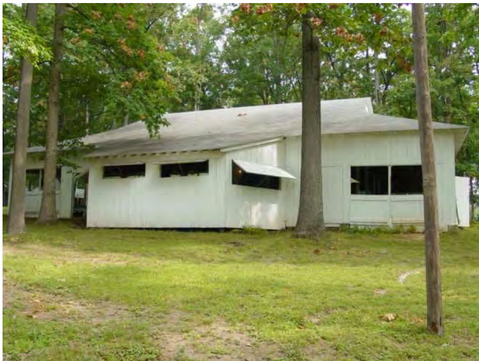
Figure VI-23: The back wall of the Spencerville tabernacle showing the projecting pulpit/choir area and the hinged window openings. (Elizabeth Jo Lampl, Montgomery County Historic Preservation Section)
