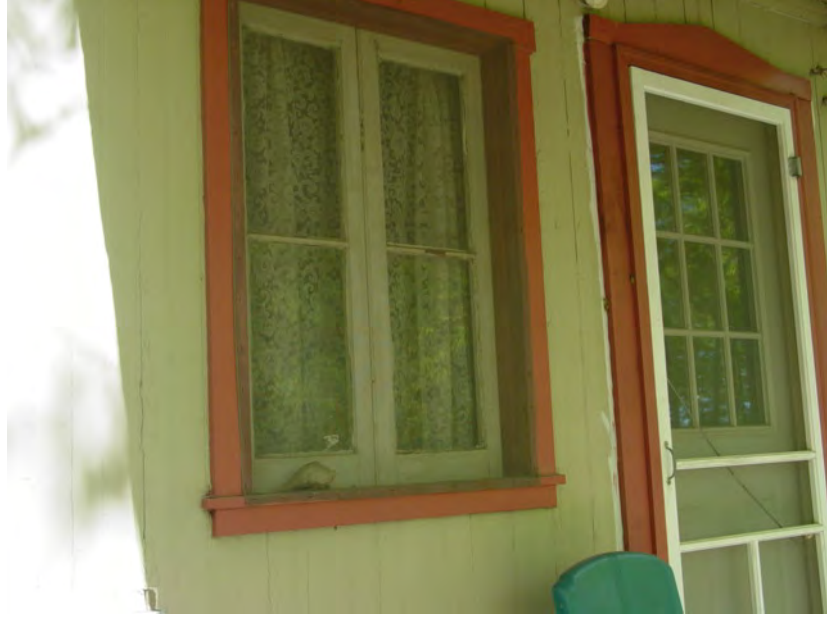
Figure VI-14: A pair of casement windows on a cottage in Spencerville. (Elizabeth Jo Lampl, Montgomery County Historic Preservation Section)
