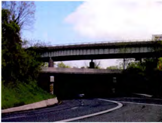
Multiple Fabricated Girders/Stringer Multi- Beam/Girder (SHA Bridge No. 0210100, MD 2 over US 50, Annapolis, MD). This is an example of multiple girders welded together.
