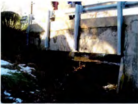
Tee Beam (SHA Bridge No. 1000600, MD 806A over High Run, Frederick County, MD)
