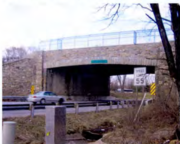
Figure 6: MD 168 over MD 295 Northbound, SHA Bridge No. 0201200 constructed in 1949 (photo by Anne Bruder, SHA, 2009)
