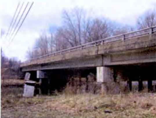
Concrete Box Beam Bridge (SHA Bridge No. 0802200, MD 225 over Mattawoman Creek, Charles County, MD)
