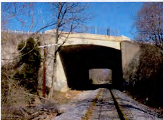
Concrete Rigid Frame (SHA Bridge No. 1010800, US 15 over Midland Railroad, Frederick County, MD)
