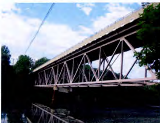
Steel Deck Truss (SHA Bridge No. 0604900, MD 26 over Liberty Reservoir, Carroll County, MD)
