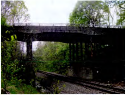
Concrete slab bridge (SHA Bridge No. 1611200, MD 381 over Norfolk Southern Railroad, Prince George's County, MD) -- the sections at the piers are haunched or deeper in order to accommodate the stress of the traffic on the deck above.
