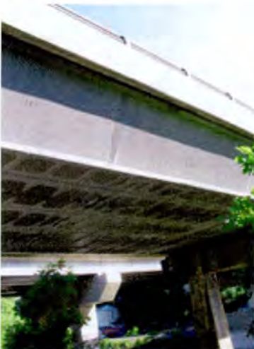
Aluminum Box Beam Bridge (SHA Bridge No. 1304600, Old MD 32 over River Road, CSX, and south Branch of Patapsco River, near Sykesville, Carroll County, MD)
