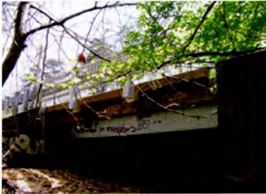
Concrete Encased Steel Beam, SHA Bridge No. 0205000, MD 176 over Piney Run, Anne Arundel County, MD
