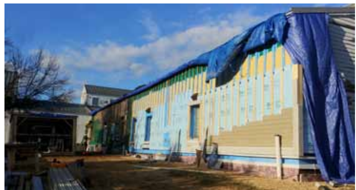
The MAC Lab is shown with its old siding removed. The building is being prepared for new siding, insulation, and roofing.
