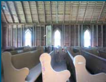
Bottom: Bazzel Church after stabilization.
