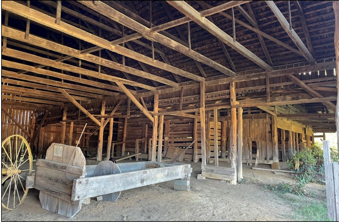
Figure 13. The Sims barn (SM-246) combines both a log crib and two types of earthfast construction. The earlier log barn, dendro-dated to 1837, was expanded within a decade by an earthfast addition with interrupted sills, then a few years later was enlarged again by the double-aisle, earthfast barn (foreground).
