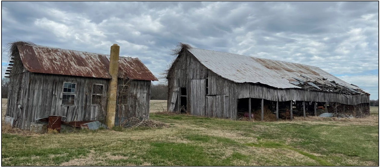
Figure 6. Albert Guy Farm, tobacco barn #2 (SM-157), with adjacent 20 th -century stripping shed; the barn and the open-sided shed have been extended in the direction of the stripping building; the original portion of the barn is in good condition, with medium integrity (facing northeast).
