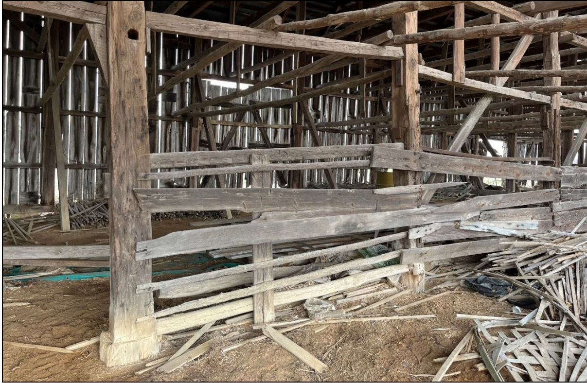
Figure 16. The Albert Guy Farm barn #2 (SM-157), hole-set posts in the foreground frame a section of one wall with continuous sills on the others.
