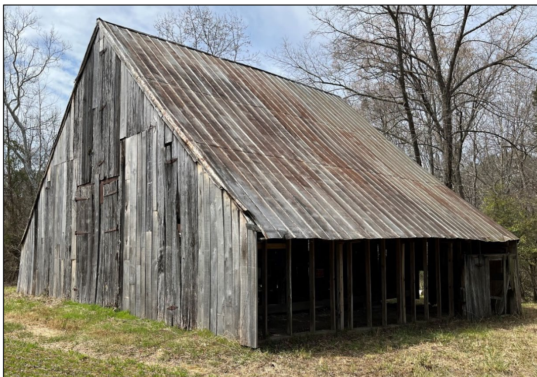
Figure 7. The remarkably well-preserved De La Brooke barn (SM-411) is representative of the early fully framed type, with two sheds (facing southwest).
