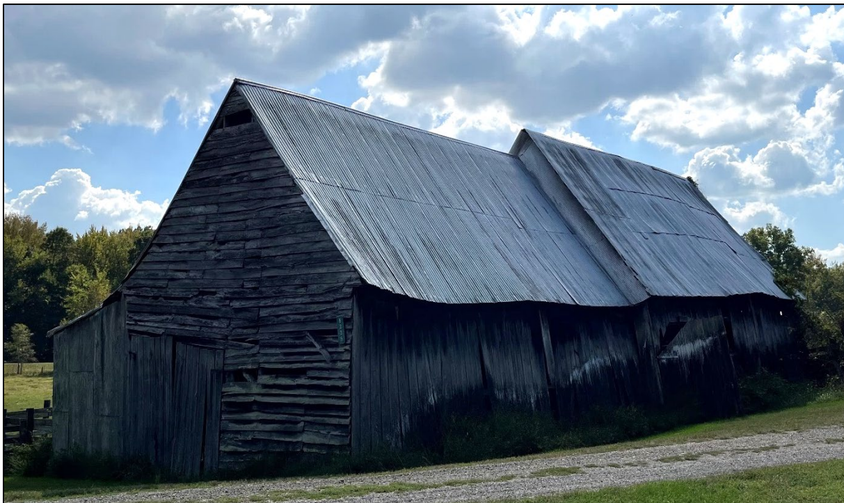
Figure 4. Plank Bridge tobacco barn (CH-174); original, earthfast section on the left; poor condition and medium integrity (facing southwest).
