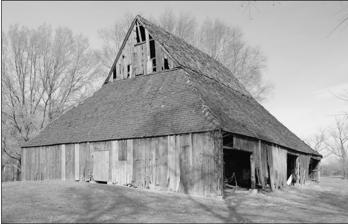
Figure 5. Warington tobacco barn (PG-733-6, HABS MD-980-1), ca. 1840s, fully framed with one original and two added sheds (non-extant).
