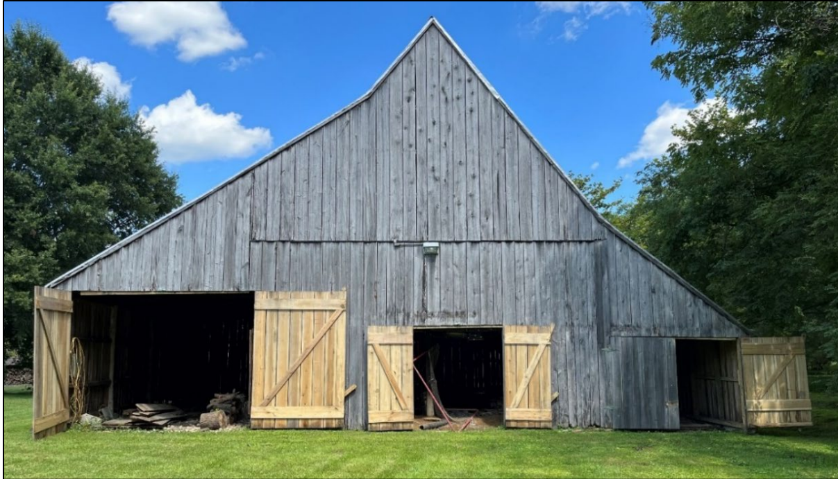
Figure 2. Tobacco barn at Rose Hill (AA-191), constructed ca. 1821; original shed on the left, early added shed on the right; the barn is in good condition and with high integrity (facing east).
