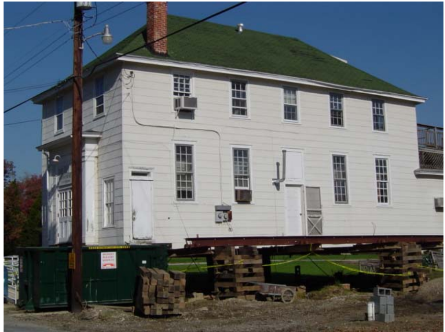
Figure 7-17 Neavitt Post Office (former Knights of Pythias lodge, early 20 th century) Hurricane Isabel damaged this structure so greatly the owner was forced to comply with flood protection codes and elevate the building. Insurance problems rife in the region after this hurricane meant a long delay in making the repairs – forcing the post office to move temporarily up the road to Bozman. To many, this post office is central to the life of the community, allowing neighbors to meet daily as they collect their mail. The tiny post offices serving country and small town populations are a character-defining feature of community life in the Stories of the Chesapeake Heritage Area. As the U. S. Postal Service seeks to keep costs down, such small offices across the nation are threatened with closure or relocation to sites out of town where shipping is easier—but no longer within reach of pedestrians. Fortunately, in Neavitt, the USPS promised to return.
