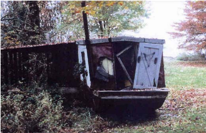
Figure 7-18 Betterton's Crownheart/Leigh Ark, c. 1886 Preservation challenges in the Stories of the Chesapeake, thanks to an extensive maritime heritage, can be a little unusual. This small houseboat is one of the last remaining vessels of its type in the Chesapeake Bay region. It was used by watermen when fishing far from home, from the 1880's to the 1920's. This particular vessel survived because it was used as an on-shore summer cottage for about thirty years in the last half of the 20 th century. The great-grandchildren of the builder have donated to the all-volunteer Betterton Community Development Corp. for its restoration.
