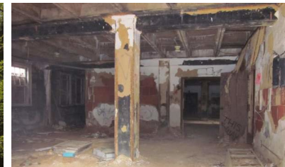
Figure 22: Interior of a building on the campus of Glenn Dale Hospital, 2016. Courtesy of M-NCPPC.
