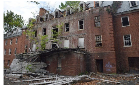
Figure 21: A building on the campus of Glenn Dale Hospital, 2015. Courtesy of Preservation Maryland.
