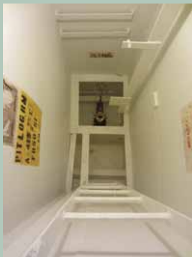
Far left: The Pit Log Room showing signs of deterioration prior to its restoration.
