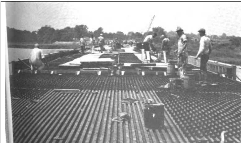
Construction photograph of the composite timber concrete bridge at Patuxent NAS published on the cover of the July 1953 issue of BuDocks Technical Digest .
