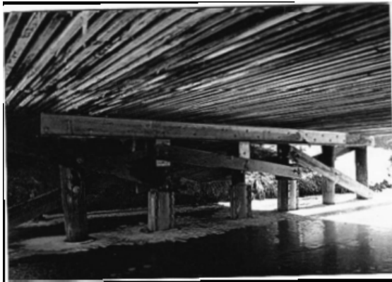
View showing composite timber and concrete deck and steel beams with pile jackets (MHT, 1998).
