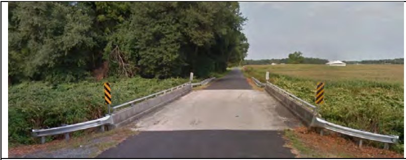
Facing northeast on Three Bridges Road towards Wicomico County Bridge WI-1231001 (Google Earth, 2014).
